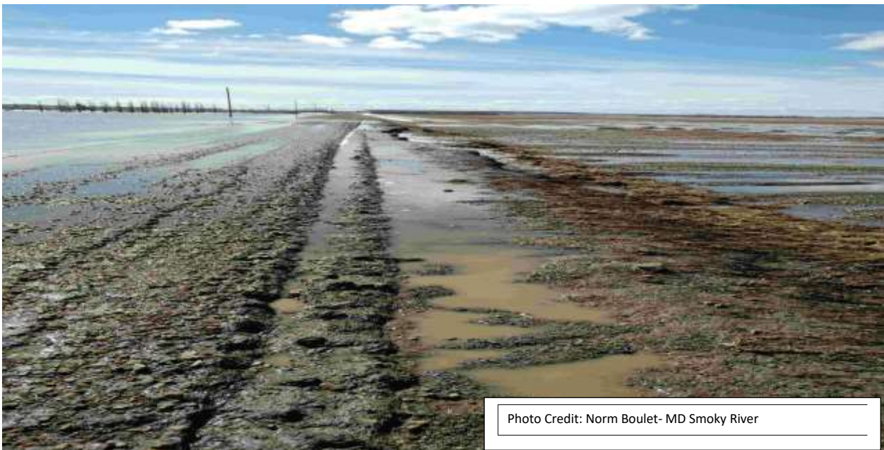
Picture 3: Road wash out due to field floods. No trees in sights
